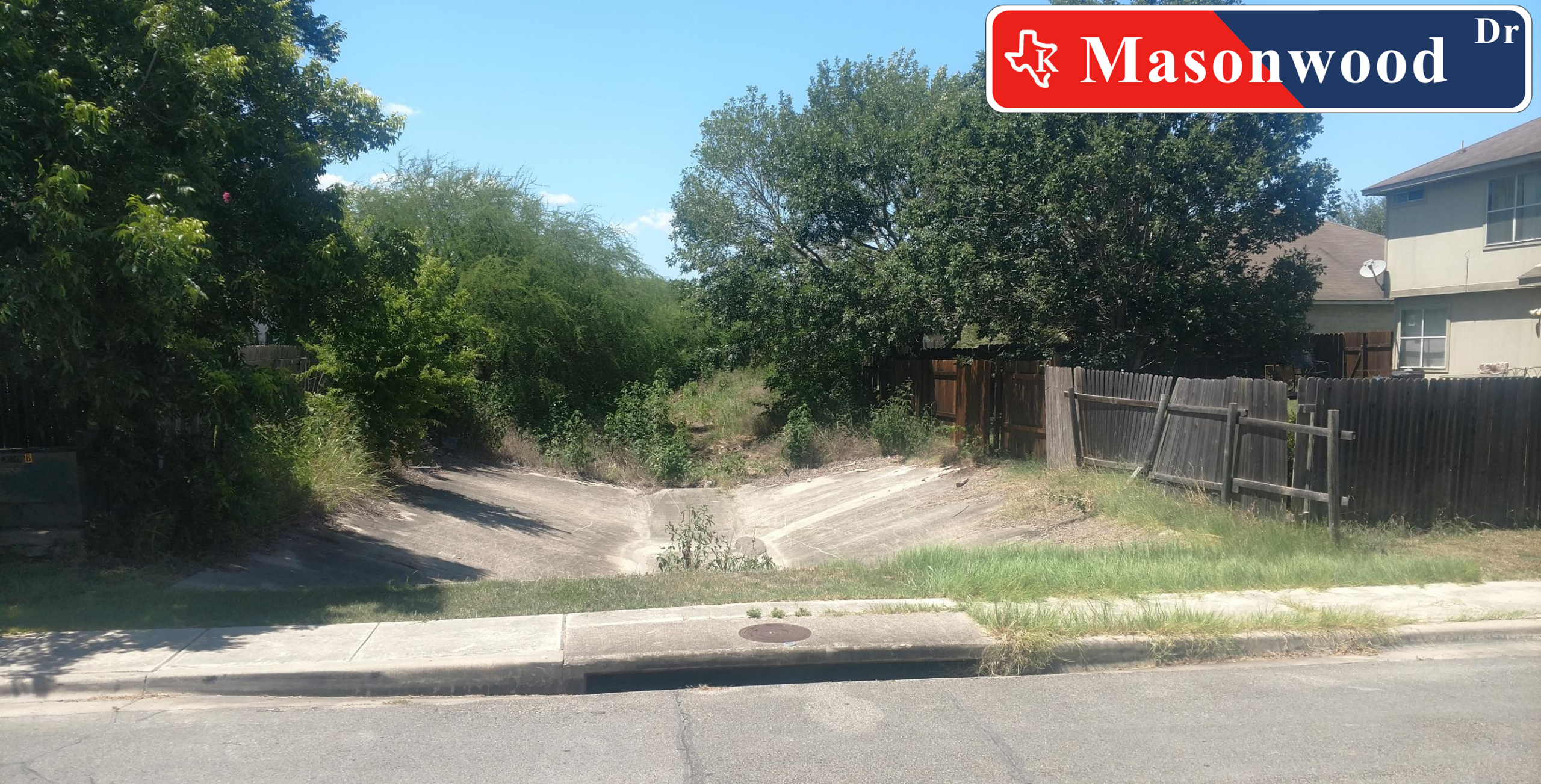
Upstream inlet at Masonwood Dr. – prior to drainage restoration 10
