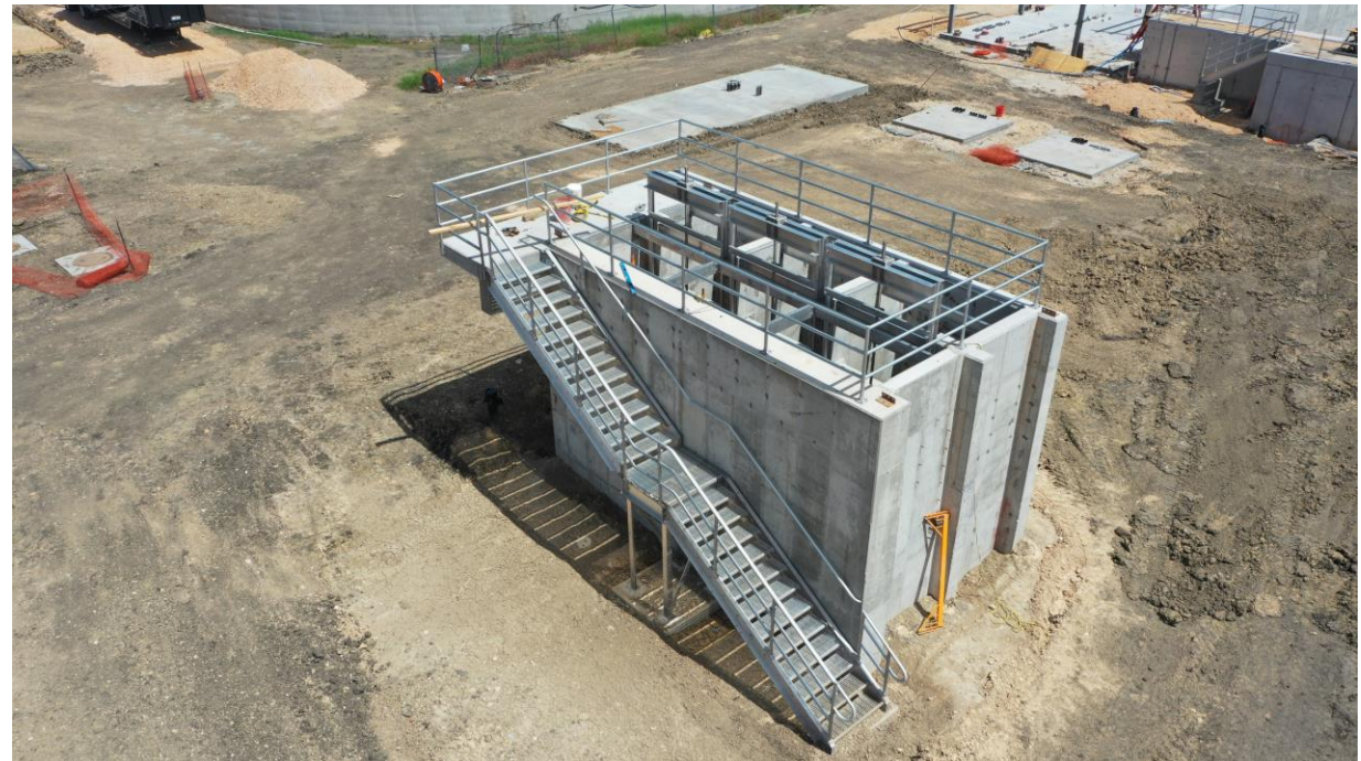
Aeration Splitter Box Stairs and Raised Gates
