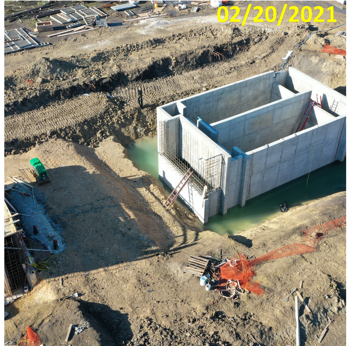
UV Disinfection Units
