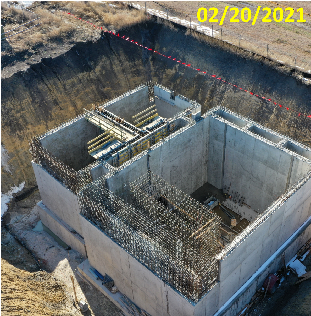
Headworks/Influent Lift Station
