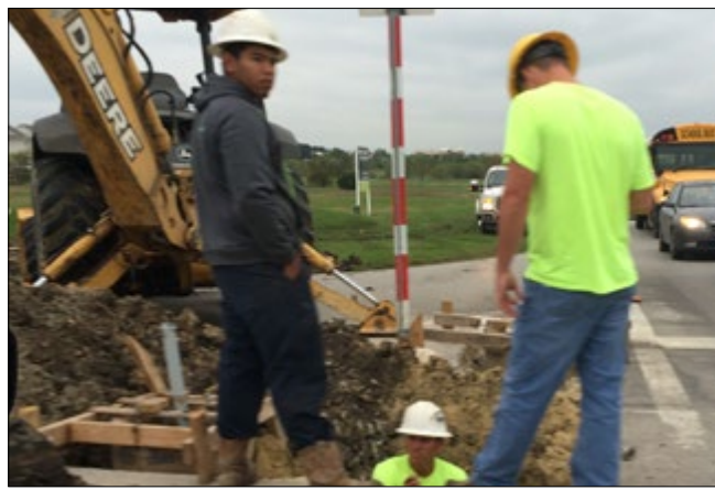
About 70 percent of underground work has been installed for the new traffic signals at FM 1626 and Kohler's Crossing.
