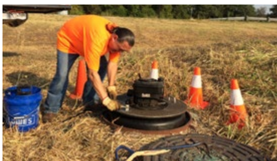
An employee from Burgess & Niple, working with Kyle's Public Works Dept., initiating a wastewater system smoke test, which finds leaks in the system.
