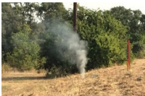
Smoke billowing up from the wastewater collection system evaluation along Old Hwy 81 in Kyle last week. Crews use smoke to test the system.
