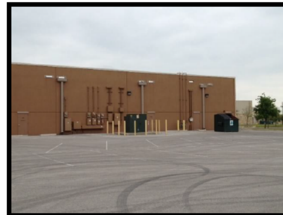
Example of unscreened utility and waste disposal areas
