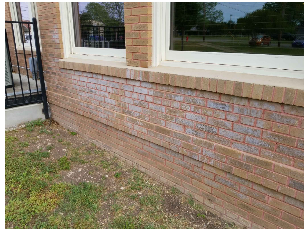
IMAGE 7: SOUTH ELEVATION: 1. EFFLORESCENCE WAS DETECTED AT THE BASE OF WALL THAT LIKELY OCCURRED DUE TO PROXIMITY OF SPRINKLERS.
