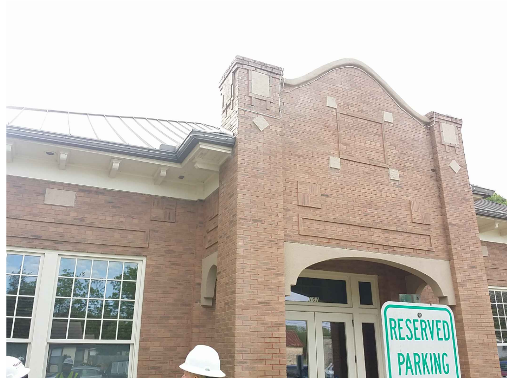
IMAGE 9: WEST ELEVATION: 1. PILASTER BRICK AND MASONRY CAP DISPLAYED SIGNIFICANT DAMAGE WITH OPEN AND FAILING MORTAR JOINTS. 2. WOOD SOFFITS ARE SAGGING AND IN SOME INSTANCES PULLING AWAY FROM ADJOINING STRUCTURE.
