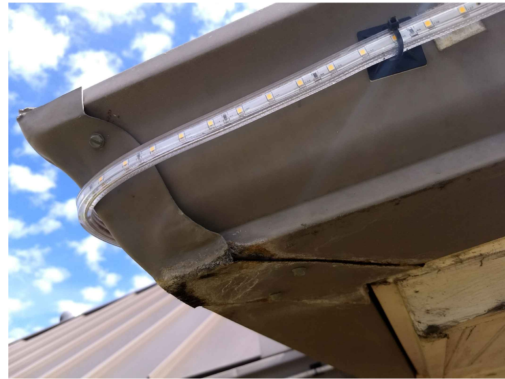
IMAGE 7: GUTTERS: DETERIORATED METAL AT SEAMS OF GUTTER.
