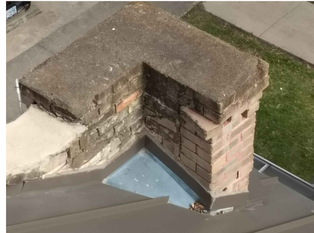
IMAGE 14: SOUTH WEST MASONRY PILASTER: 1. PILASTER BRICK AND MASONRY CAP DISPLAYED SIGNIFICANT DAMAGE WITH OPEN AND FAILING MORTAR JOINTS.
