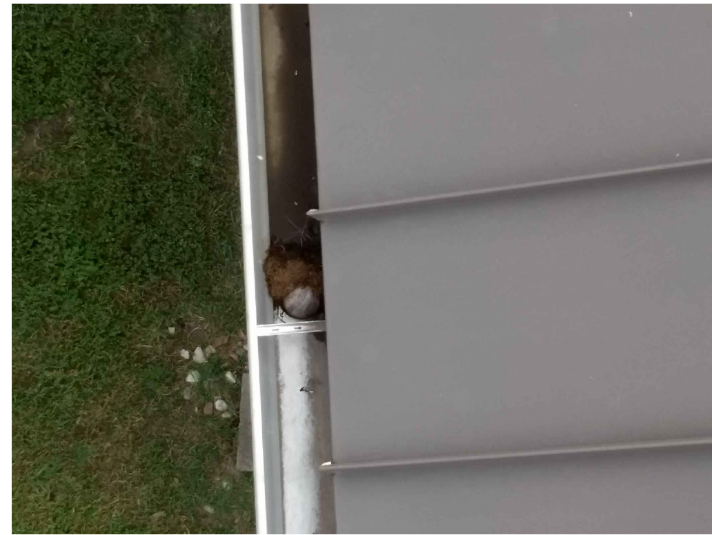
IMAGE 6: GUTTERS: EXCESSIVE DEBRIS IN THE GUTTER OBSTRUCTING GUTTERS AND DOWNSPOUTS MAY CONTRIBUTE TO GUTTER OVERFLOW.
