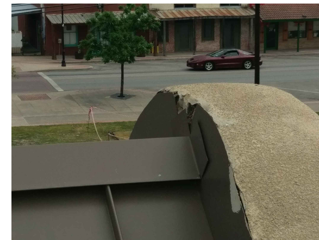
IMAGE 12: ARCH OVER ENTRYWAYS: SEVERAL AREAS AT ALL LOCATIONS SHOW DETERIORATION AT THE EDGE OF THE CEMENT WASH AND OPENINGS AT THE INTERSECTION OF THE SHEET METAL FLASHINGS. ALSO, SIGNIFICANT DETERIORATION OF THE ADJOINING MASONRY, ALLOWING AN ENTRY POINT FOR MOISTURE.
