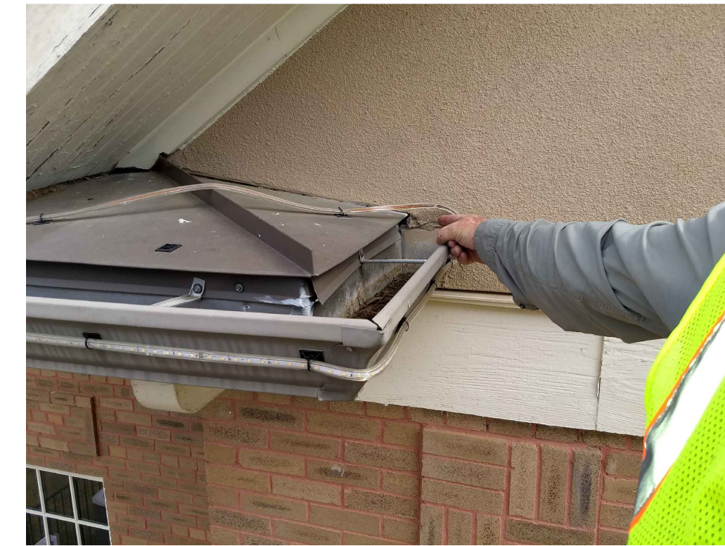
IMAGE 8: STUCCO: HOLE IN STUCCO AT TRANSITION FROM METAL ROOF TO STUCCO ALLOWS WATER INTO EXTERIOR WALL CONSTRUCTION.
