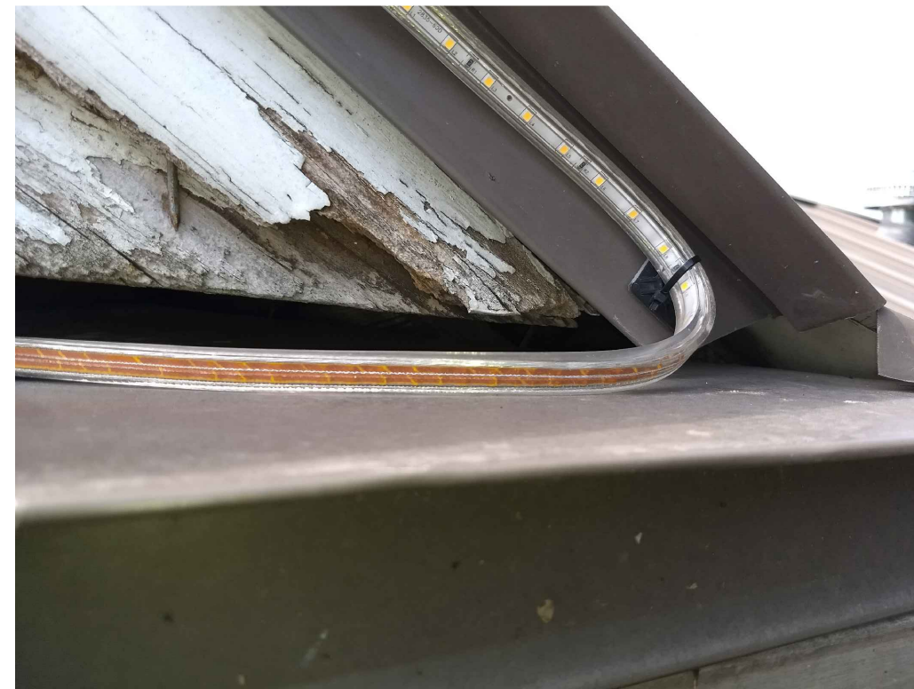
IMAGE 5: WOOD: SOFFITS SAGGING AND PULLING AWAY FROM THE STRUCTURE. DETERIORATION OF WOOD COMPONENTS AND STRUCTURAL THERMAL MOVEMENT HAVE RESULTED IN LOSS OF POSITIVE SECUREMENT OF THESE SOFFIT ASSEMBLIES WHICH IS A SAFETY CONCERN.
