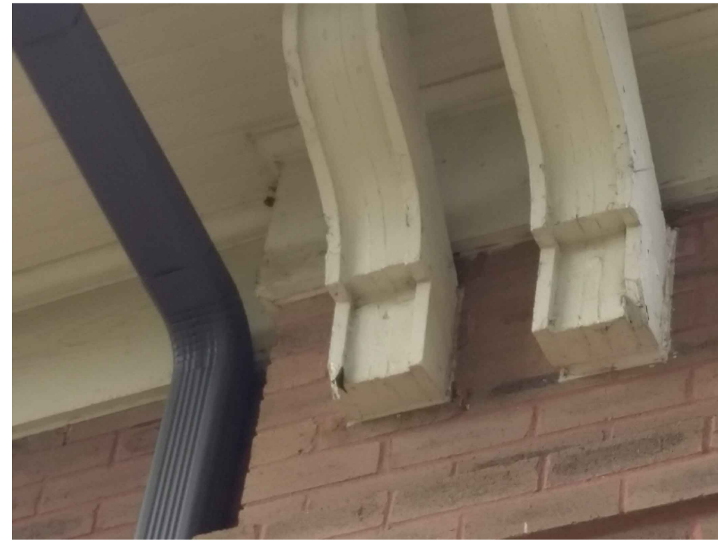
IMAGE 1: WOOD: CHIPPING PAINT ON SOFFIT AND SOFFIT ORNAMENTAL ELEMENTS.
