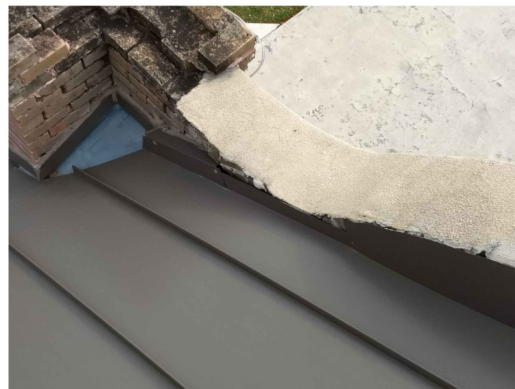
IMAGE 9: ARCH OVER ENTRYWAYS: SEVERAL AREAS AT ALL LOCATIONS SHOW DETERIORATION AT THE EDGE OF THE CEMENT WASH AND OPENINGS AT THE INTERSECTION OF THE SHEET METAL FLASHINGS. ALSO, SIGNIFICANT DETERIORATION OF THE ADJOINING MASONRY, ALLOWING AN ENTRY POINT FOR MOISTURE.
