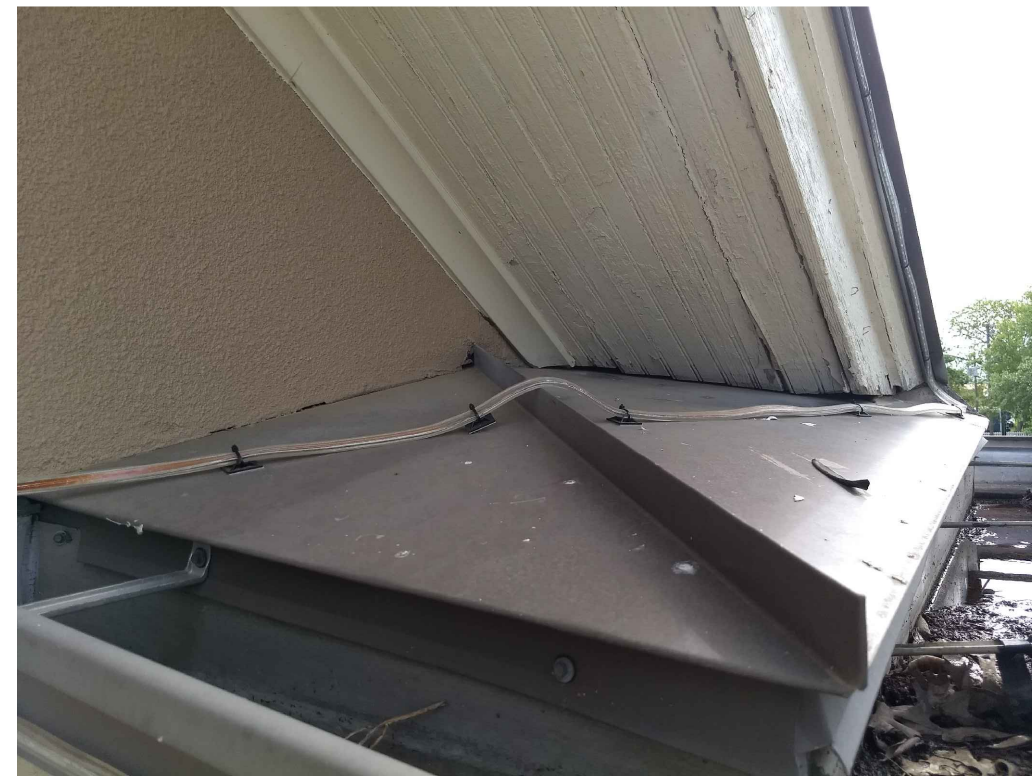
IMAGE 6: WOOD: SOFFITS SAGGING AND PULLING AWAY FROM THE STRUCTURE. DETERIORATION OF WOOD COMPONENTS AND STRUCTURAL THERMAL MOVEMENT HAVE RESULTED IN LOSS OF POSITIVE SECUREMENT OF THESE SOFFIT ASSEMBLIES WHICH IS A SAFETY CONCERN.
