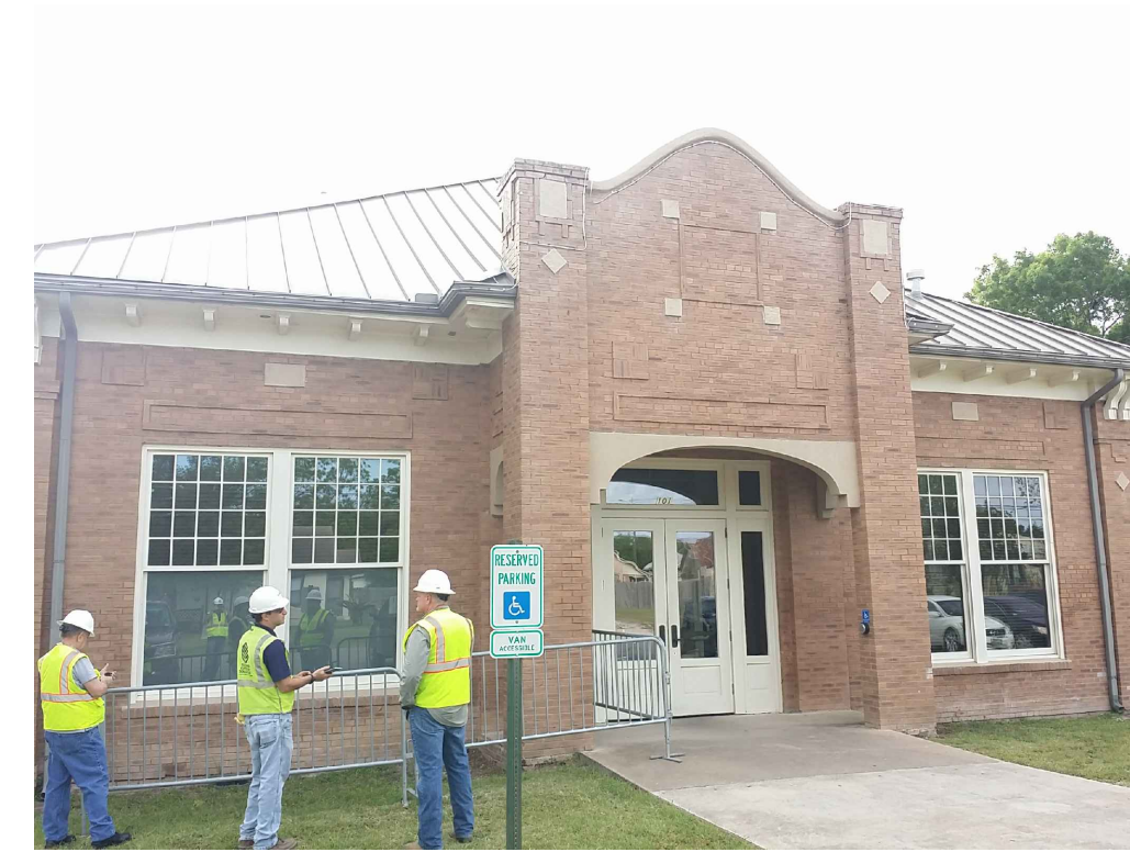
IMAGE 4: WEST ELEVATION: 1. EFFLORESCENCE WAS DETECTED AT THE BASE OF WALL THAT LIKELY OCCURRED DUE TO PROXIMITY OF SPRINKLERS. 2. PILASTER BRICK AND MASONRY CAP DISPLAYED SIGNIFICANT DAMAGE WITH OPEN AND FAILING MORTAR JOINTS. 3. WOOD SOFFITS ARE SAGGING AND IN SOME INSTANCES PULLING AWAY FROM ADJOINING STRUCTURE.
