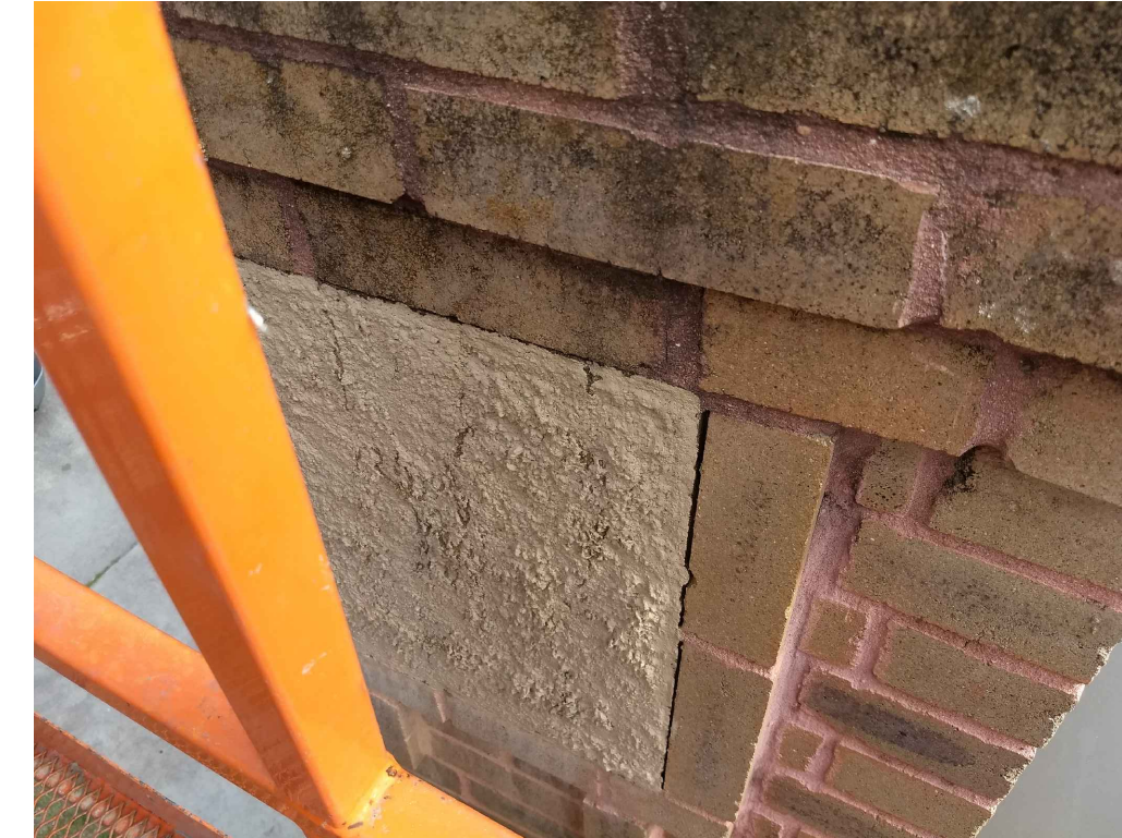
IMAGE 12: TYPICAL STUCCO TO BRICK TRANSITION: SEPARATION AT JOINT BETWEEN STUCCO AND BRICK.
