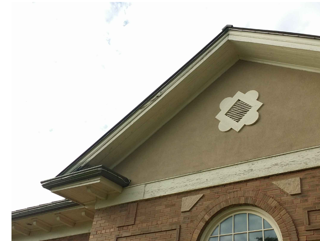
IMAGE 8: WOOD: WOOD SOFFIT AND FASCIA DETERIORATION SEAM INCONSISTENT WITH THE RECENT METAL ROOF INSTALLATION, INDICATING THE EXISTING SOFFITS AND FASCIA WERE NOT REPLACED RECENTLY BUT LIKELY REPAINTED. IN ISOLATED INSTANCES FAILURE DUE TO THE GUTTER SEAMS HAS CONTRIBUTED TO THE DETERIORATION.
