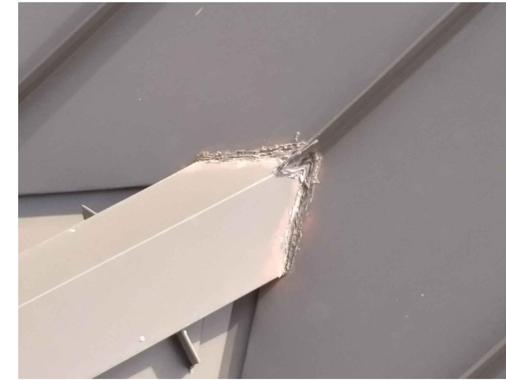
IMAGE 4: ROOF: DETERIORATING SEALANT WAS NOTED AT THE INTERSECTION OF THE METAL ROOF PANELS TO DORMERS. THE INTERSECTION OF DORMER ROOF TO THE METAL ROOF PANELS DOES NOT HAVE A FLASHING AND INSTEAD RELIES ON SEALANT TO MAINTAIN A WATER TIGHT INTERSECTION.
