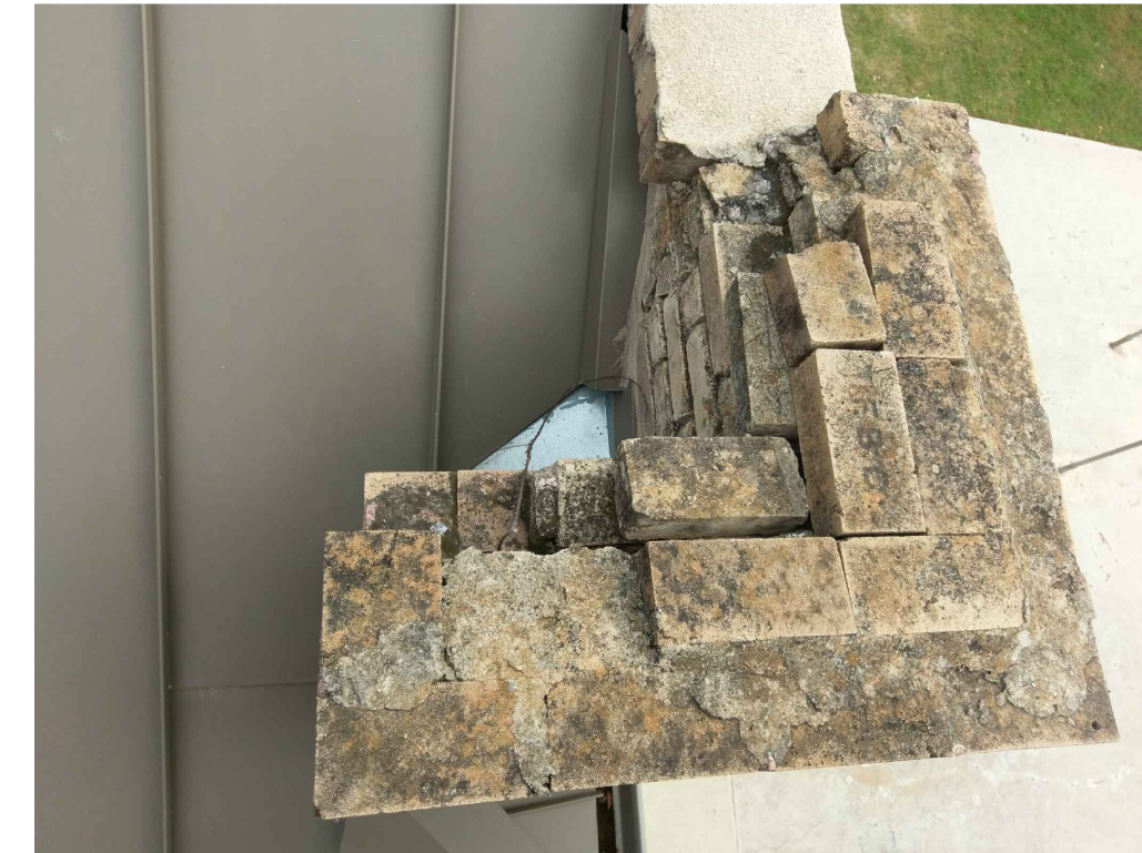
IMAGE 16: SOUTH EAST MASONRY PILASTER: 1. PILASTER BRICK AND MASONRY CAP DISPLAYED SIGNIFICANT DAMAGE WITH OPEN AND FAILING MORTAR JOINTS AND LOOSE SHIFTING BRICKS.
