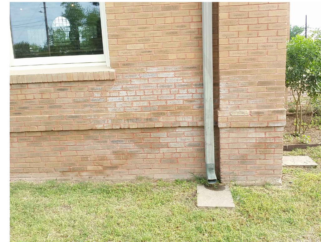
IMAGE 8: SOUTH ELEVATION: 1. EFFLORESCENCE WAS DETECTED AT THE BASE OF WALL THAT LIKELY OCCURRED DUE TO PROXIMITY OF SPRINKLERS.
