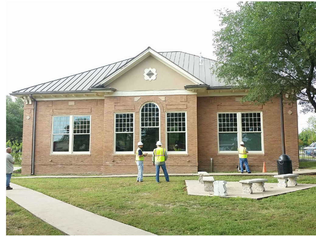
IMAGE 2: NORTH ELEVATION: 1. EFFLORESCENCE WAS DETECTED AT THE BASE OF WALL THAT LIKELY OCCURRED DUE TO PROXIMITY OF SPRINKLERS. 2. WOOD SOFFITS ARE SAGGING AND IN SOME INSTANCES PULLING AWAY FROM ADJOINING STRUCTURE. 3. DETERIORATION OF WOOD FASCIA. 4. DETERIORATION OF FASCIA RESULTING IN LOCALIZED SEPARATION OF THE GUTTER ASSEMBLY.
