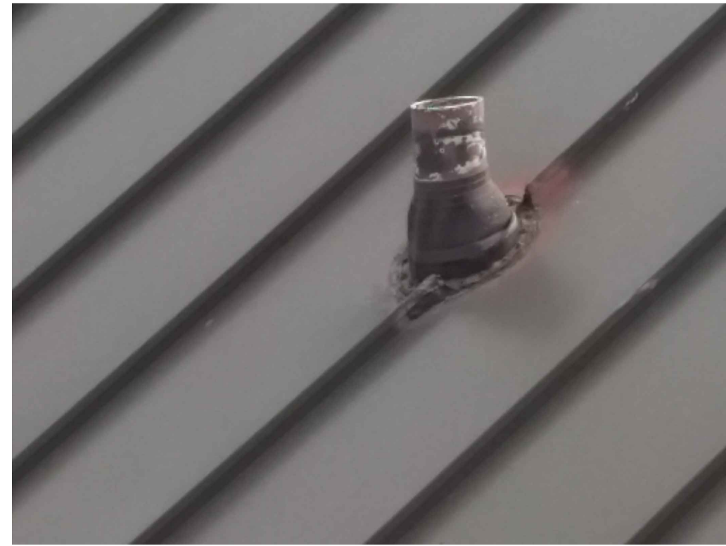
IMAGE 3: ROOF: EXISTING SEALANT IS TEMPORARY SEALANT.
