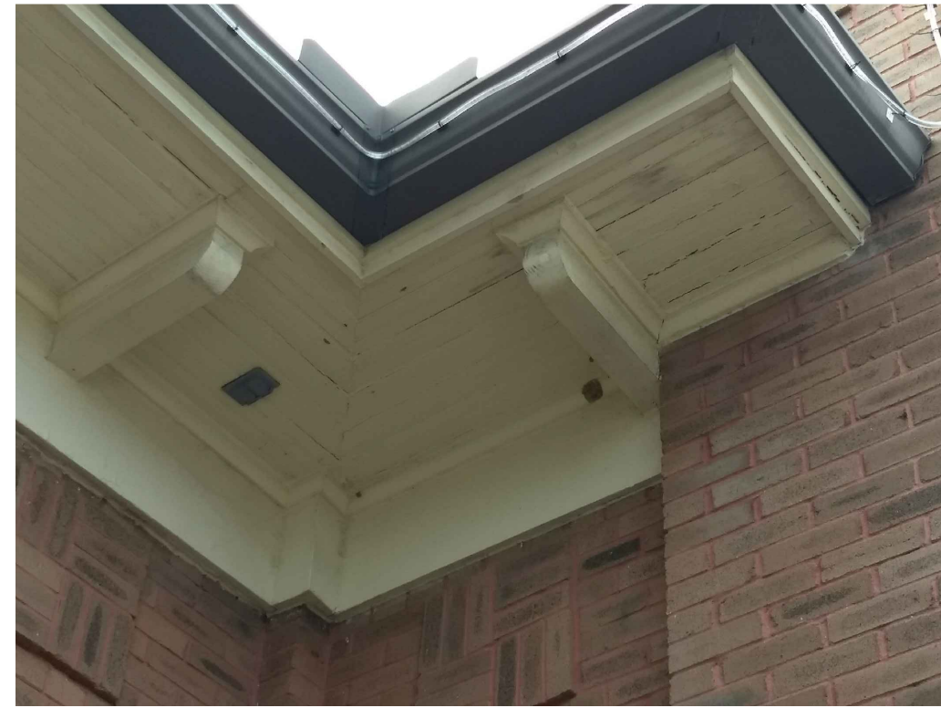
IMAGE 2: WOOD: SOFFITS SAGGING AND PULLING AWAY FROM THE STRUCTURE. DETERIORATION AT THE TOP OF THE ENTRANCE WAY MASONRY IS RESULTING IN WATER ENTRY IN THESE AREAS, CONTRIBUTING TO VISIBLE DAMAGE TO WOOD FASCIA AND SOFFIT ASSEMBLIES AND LIKELY DAMAGE TO UNDERLYING WOOD DECK AND SUPPORT MEMBERS.
