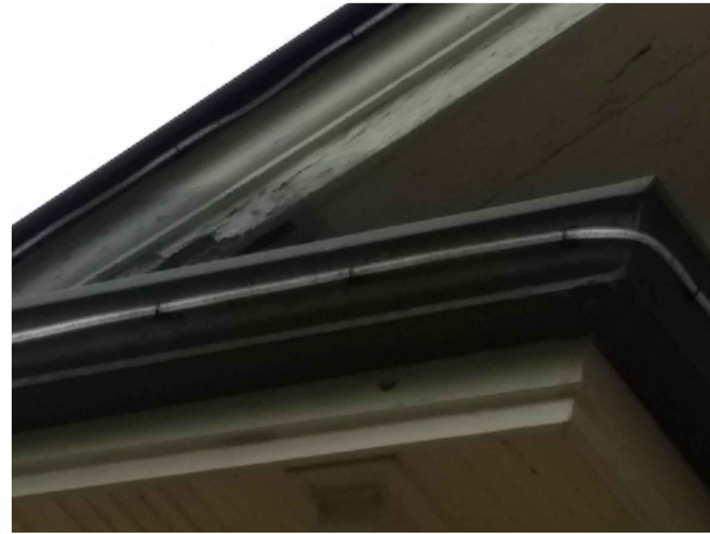
IMAGE 2: WOOD: SOFFITS SAGGING AND PULLING AWAY FROM THE STRUCTURE. DETERIORATION AT THE TOP OF THE ENTRANCE WAY MASONRY IS RESULTING IN WATER ENTRY IN THESE AREAS, CONTRIBUTING TO VISIBLE DAMAGE TO WOOD FASCIA AND SOFFIT ASSEMBLIES AND LIKELY DAMAGE TO UNDERLYING WOOD DECK AND SUPPORT MEMBERS.
