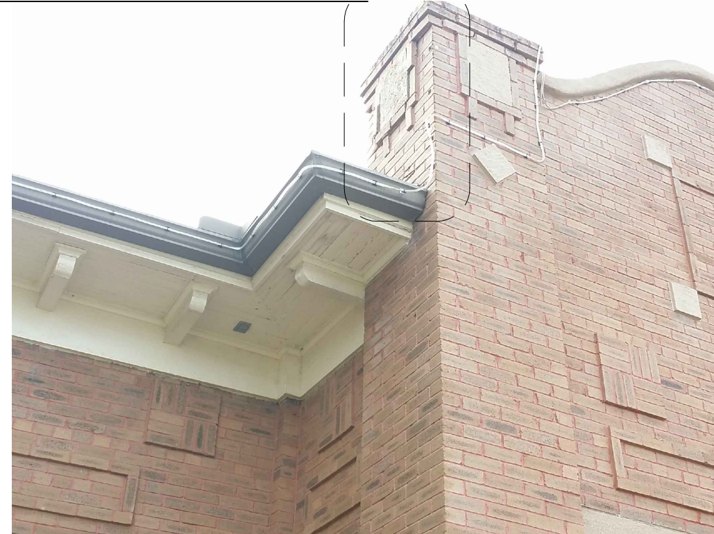
IMAGE 11: WEST ELEVATION: 1. PILASTER BRICK AND MASONRY CAP DISPLAYED SIGNIFICANT DAMAGE WITH OPEN AND FAILING MORTAR JOINTS. 2. WOOD SOFFITS ARE SAGGING AND IN SOME INSTANCES PULLING AWAY FROM ADJOINING STRUCTURE.
