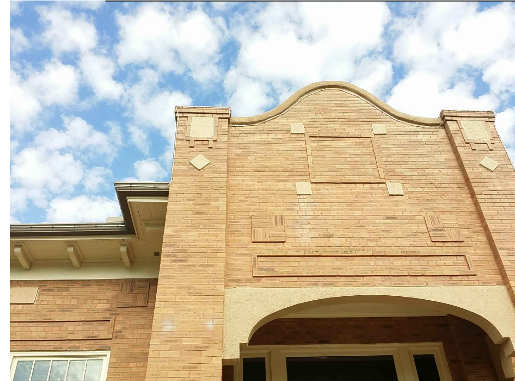
IMAGE 10: EAST ELEVATION: 1. PILASTER BRICK AND MASONRY CAP DISPLAYED SIGNIFICANT DAMAGE WITH OPEN AND FAILING MORTAR JOINTS. 2. WOOD SOFFITS ARE SAGGING AND IN SOME INSTANCES PULLING AWAY FROM ADJOINING STRUCTURE.
