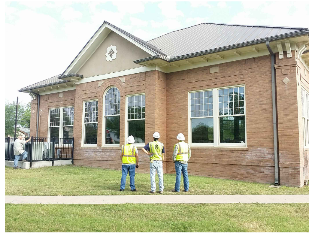
IMAGE 3: SOUTH ELEVATION: 1. EFFLORESCENCE WAS DETECTED AT THE BASE OF WALL THAT LIKELY OCCURRED DUE TO PROXIMITY OF SPRINKLERS. 2. WOOD SOFFITS ARE SAGGING AND IN SOME INSTANCES PULLING AWAY FROM ADJOINING STRUCTURE. 3. DETERIORATION OF WOOD FASCIA. 4. DETERIORATION OF FASCIA RESULTING IN LOCALIZED SEPARATION OF THE GUTTER ASSEMBLY.
