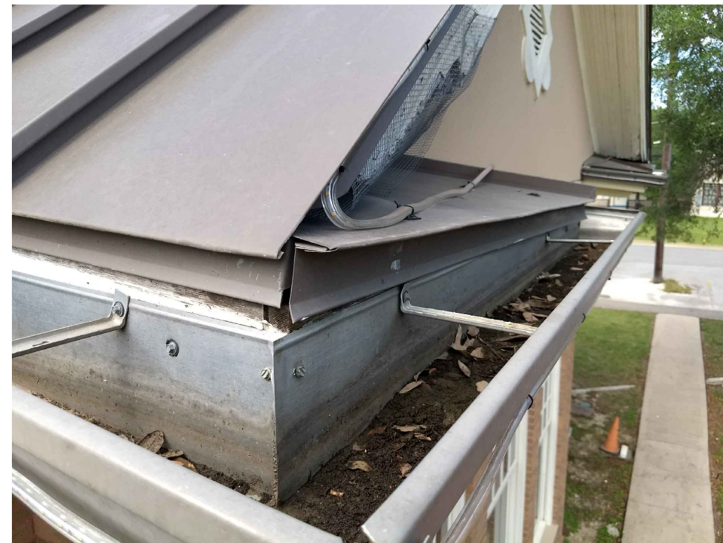
IMAGE 7: WOOD: SOFFITS SAGGING AND PULLING AWAY FROM THE STRUCTURE. GUTTERS WATER GETTING BACKED UP IN THE GUTTER DUE TO DEBRIS BLOCKING THE DOWNSPOUTS IS BACKING INTO THE OVERHANG STRUCTURE IS BELIEVED TO BE CAUSING DAMAGE TO FASCIA AND SOFFITS.
