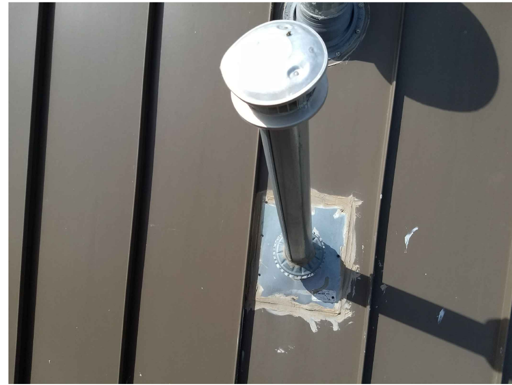
IMAGE 2: ROOF: VENT AND PLUMBING PENETRATIONS THROUGH THE METAL ROOF WERE IN FUNCTIONAL CONDITION WITH THE EXCEPTION OF THE VENT PIPE ASSOCIATED WITH THE WATER HEATER AND INTERIOR LEAK. EXPOSED FASTENERS AND TEMPORARY SEALANT AT THE HOT WATER VENT STACK PENETRATION.
