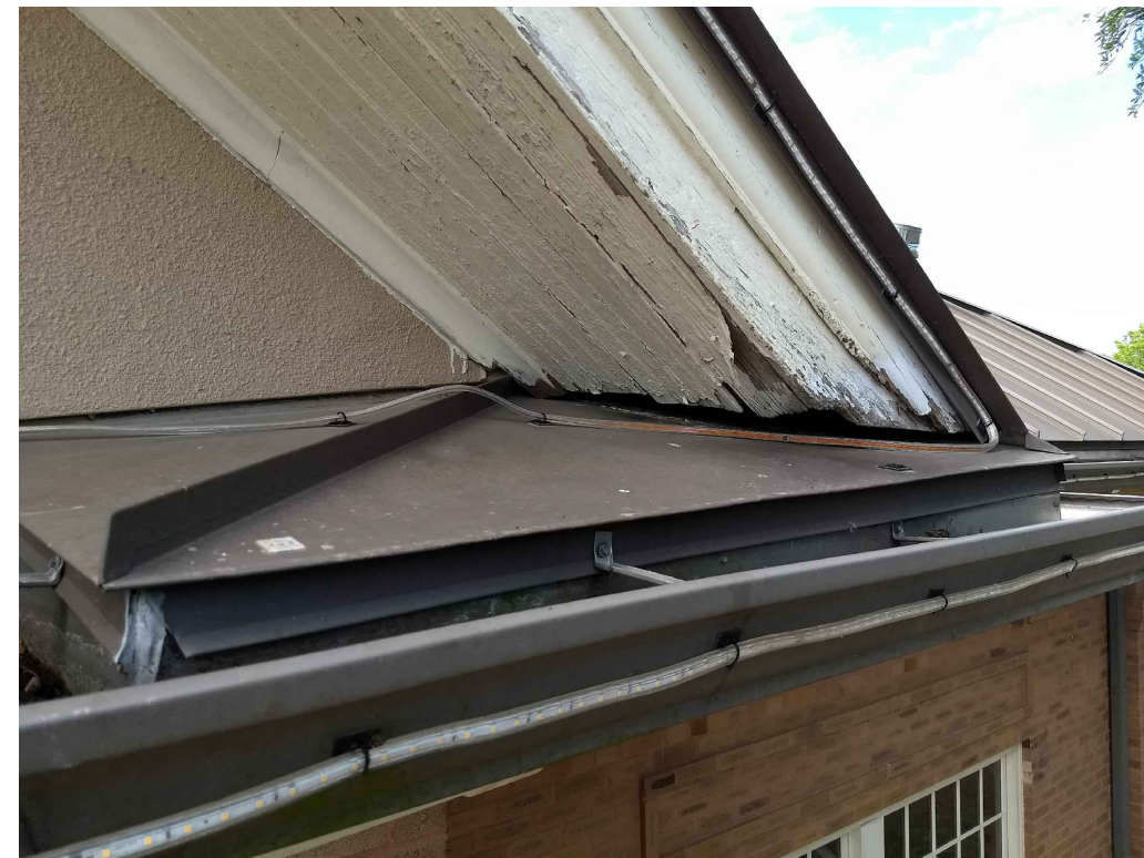
IMAGE 11: WOOD SOFFIT AND FASCIA DETERIORATION SEAM INCONSISTENT WITH THE RECENT METAL ROOF INSTALLATION, INDICATING THE EXISTING SOFFITS AND FASCIA WERE NOT REPLACED RECENTLY BUT LIKELY REPAINTED. IN ISOLATED INSTANCES FAILURE DUE TO THE GUTTER SEAMS HAS CONTRIBUTED TO THE DETERIORATION.
