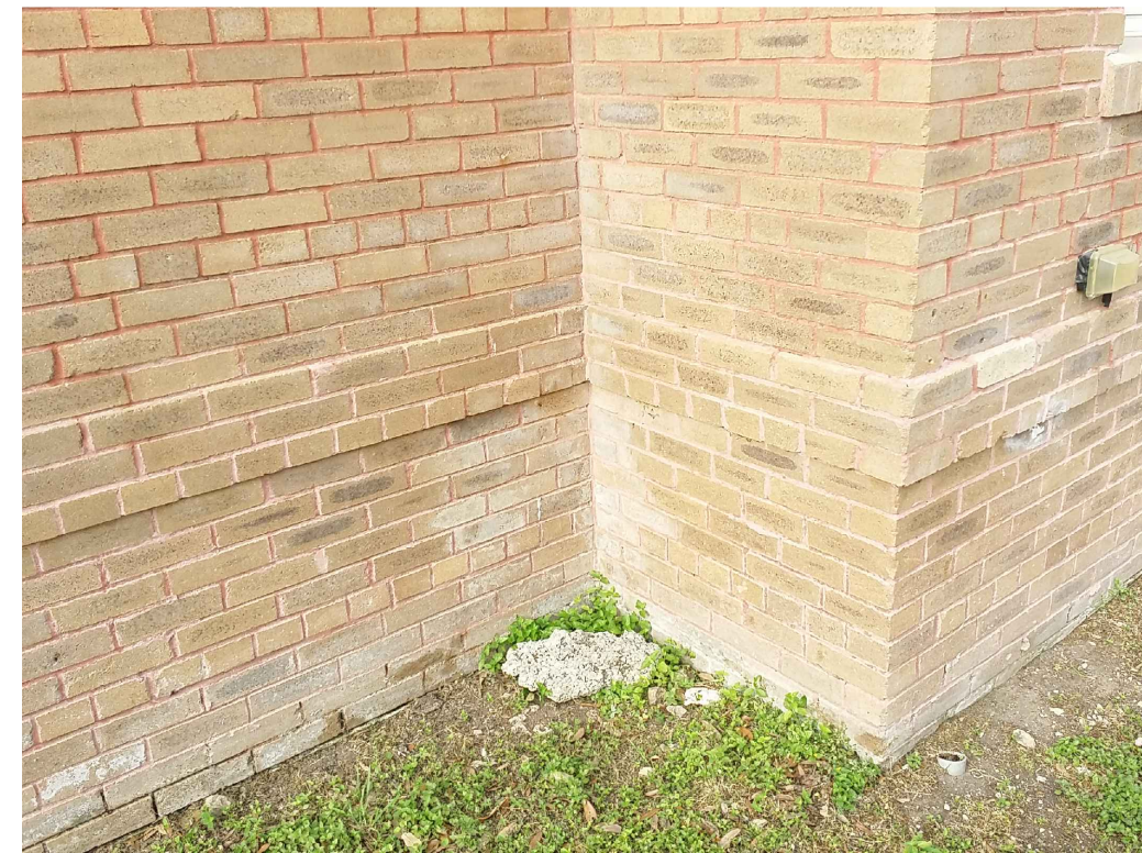
IMAGE 6: NORTH ELEVATION: 1. EFFLORESCENCE WAS DETECTED AT THE BASE OF WALL THAT LIKELY OCCURRED DUE TO PROXIMITY OF SPRINKLERS.
