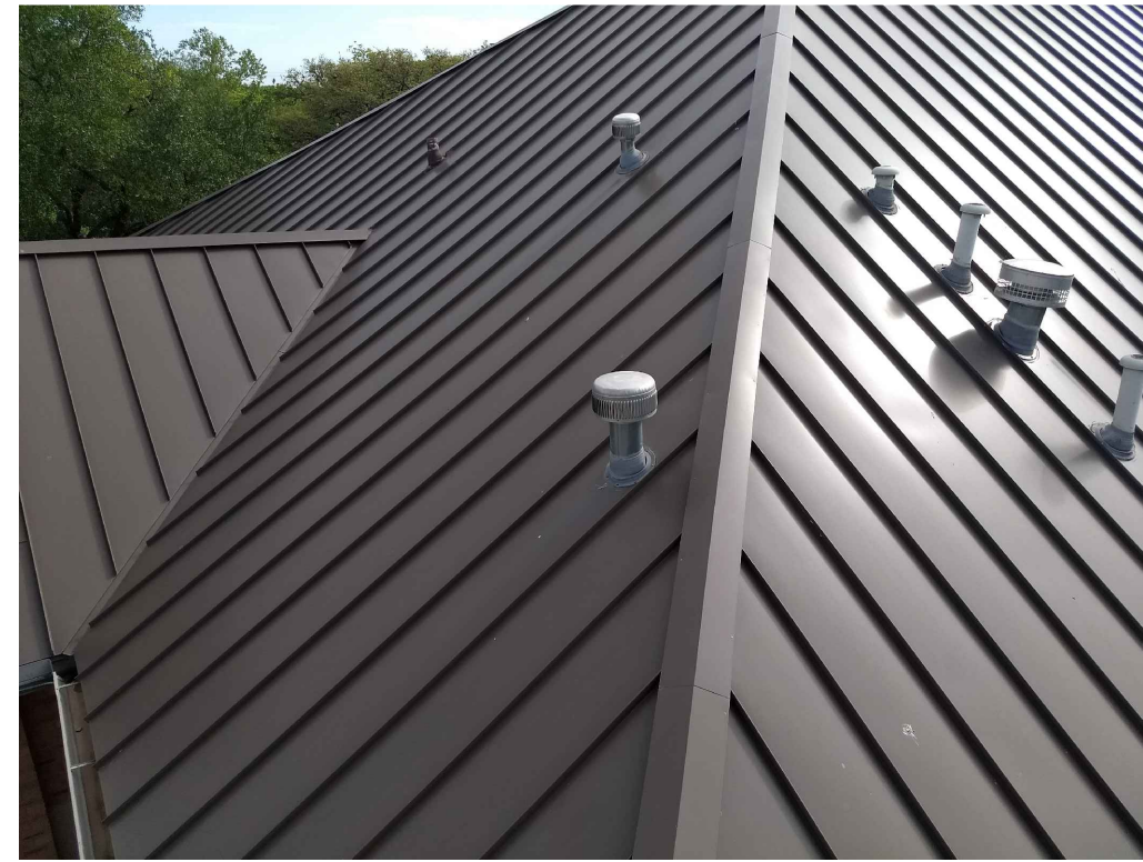
IMAGE 1: ROOF: VENT AND PLUMBING PENETRATIONS THROUGH THE METAL ROOF WERE IN FUNCTIONAL CONDITION WITH THE EXCEPTION OF THE VENT PIPE ASSOCIATED WITH THE WATER HEATER AND INTERIOR LEAK. EXPOSED FASTENERS AND TEMPORARY SEALANT AT THE HOT WATER VENT STACK PENETRATION.
