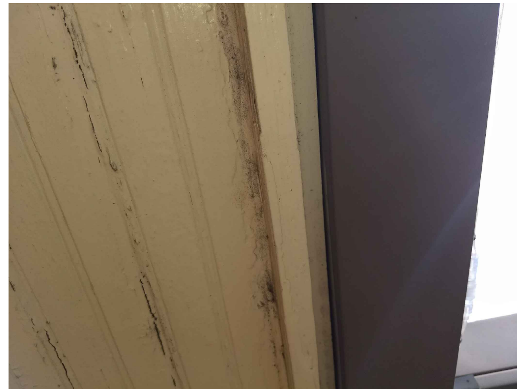
IMAGE 9: WOOD: SOFFITS SAGGING AND PULLING AWAY FROM THE STRUCTURE. DEBRIS OBSTRUCTING THE GUTTER AND DOWNSPOUTS MAY CONTRIBUTE TO GUTTER OVERFLOW DURING RAIN EVENTS.
