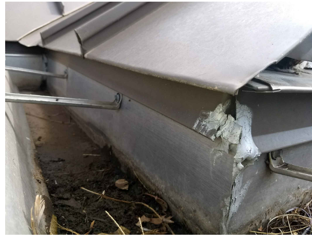
IMAGE 5: GUTTERS: GUTTER ASSEMBLY HAS LOST SECUREMENT TO THE WOOD FASCIA. DETERIORATED WOOD FASCIA AND COMPONENTS ARE NO LONGER PROVIDING SECURE AND SAFE SUBSTRATE FOR THE ATTCHMENT OF GUTTER ASSEMBLY.
