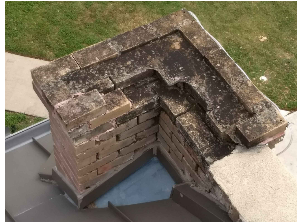
IMAGE 15: NORTH EAST MASONRY PILASTER: 1. PILASTER BRICK AND MASONRY CAP DISPLAYED SIGNIFICANT DAMAGE WITH OPEN AND FAILING MORTAR JOINTS.
