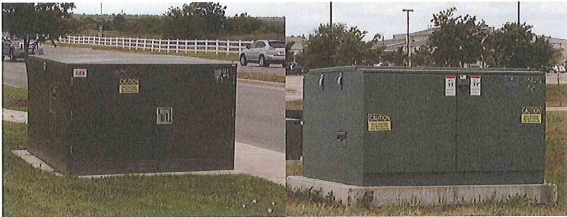
Switchgear Boxes (for visual comparison to the below option)
