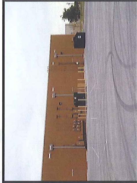
Example of unscreened utility and waste disposal areas
