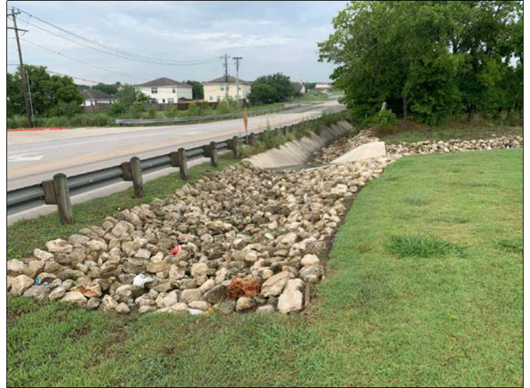
22. Looking west along roadside ditch towards Richmond Branch. Riprap has been installed to minimize erosion.
