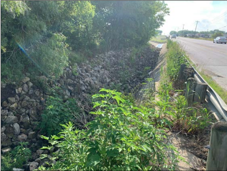
25. Looking east along roadside ditch near the discharge point into Richmond Branch. Significant riprap has been installed to minimize erosion.
