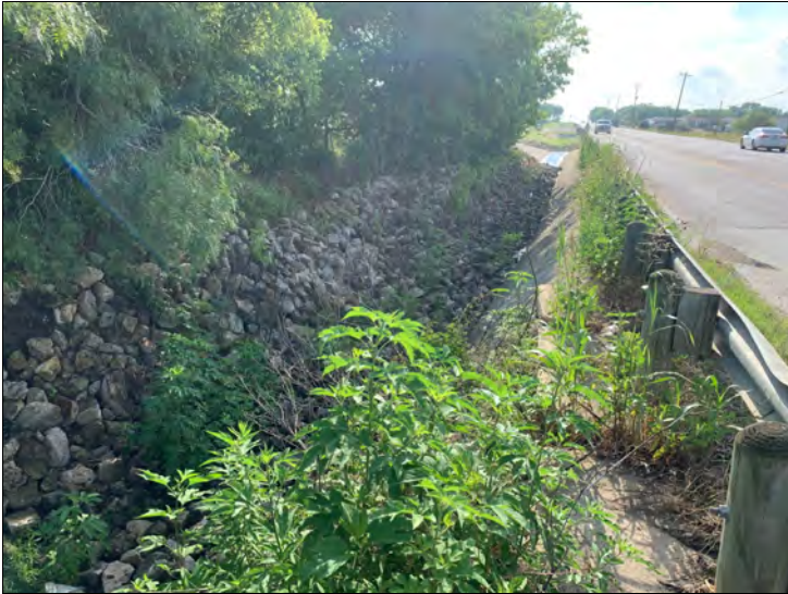
25. Looking east along roadside ditch near the discharge point into Richmond Branch. Significant riprap has been installed to minimize erosion.
