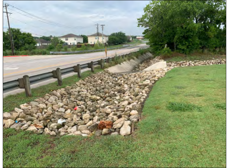
22. Looking west along roadside ditch towards Richmond Branch. Riprap has been installed to minimize erosion.
