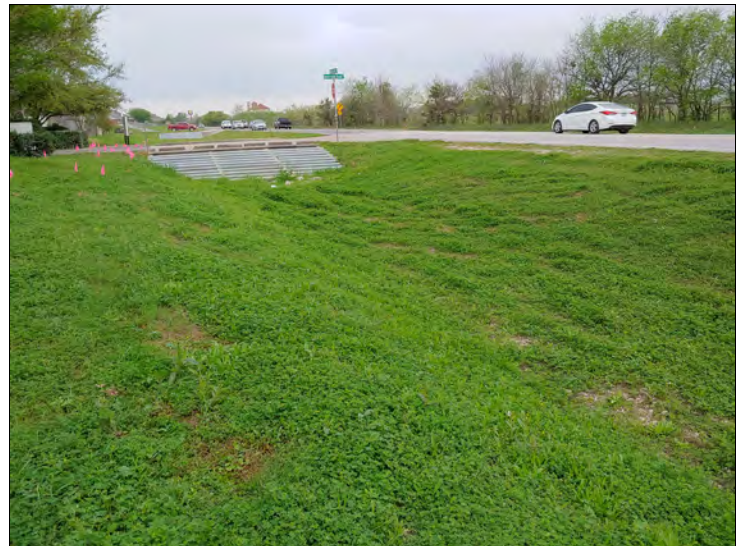
12. For comparison: Photograph taken by FLT in March 2020 showing typical, dry conditions of the roadside ditch.
