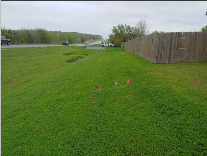
7. For comparison: Photograph taken by FLT in March 2020 showing typical, dry site conditions of the roadside ditch.
