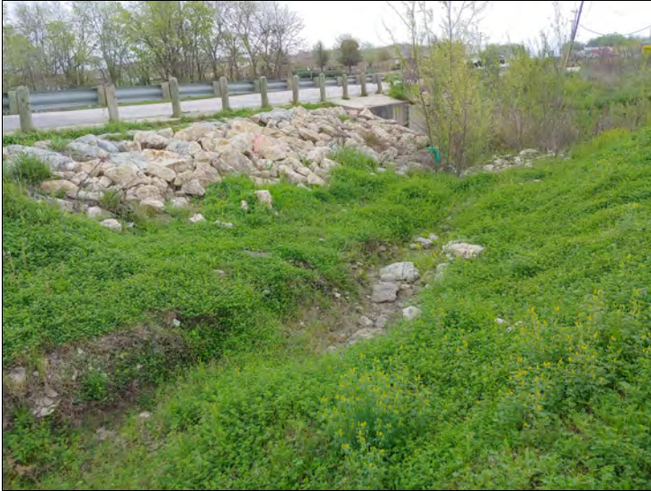
15. Looking east along roadside ditch near Richmond Branch bridge. Significant erosion is present, along with erosion control devices put in place over the years.
