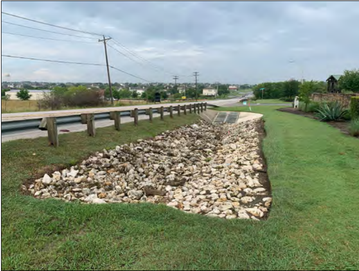
19. Looking west along the north roadside ditch near Purple Martin Ave. Riprap has been installed to minimize erosion.
