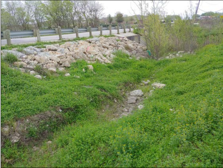
15. Looking east along roadside ditch near Richmond Branch bridge. Significant erosion is present, along with erosion control devices put in place over the years.
