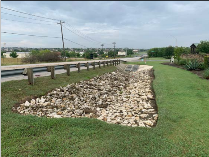
19. Looking west along the north roadside ditch near Purple Martin Ave. Riprap has been installed to minimize erosion.
