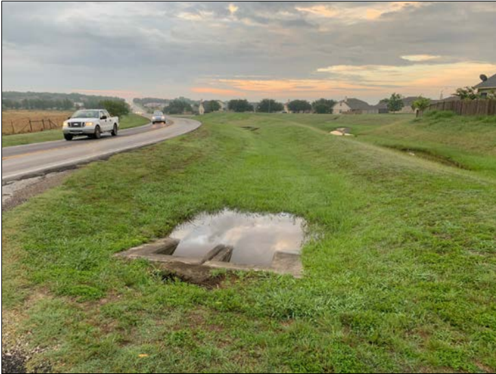
1. Looking east along Windy Hill Road and the south roadside ditch during the June 2020 delineation.
