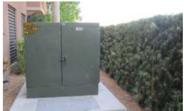
Hedge screening Transformer Box with adequate space between landscaping and box for maintenance
