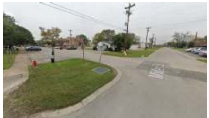
Example of Inaccessible conditions; lack of textured wheelchair ramps on each side of the street corner, and sidewalk is disconnected from street crossing, with no sidewalk on the other side of the road; lack of a clear crosswalk
