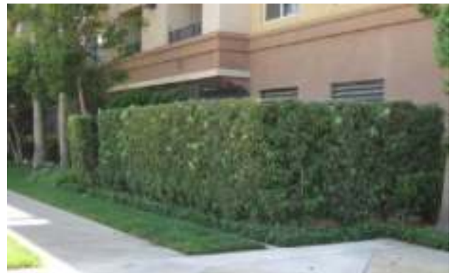
Hedge screening Transformer Box from view
